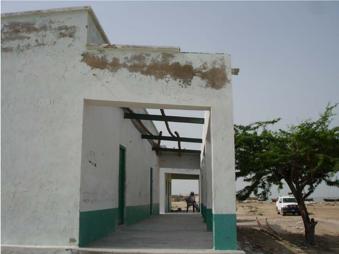
Figure 4: Blew away roof top of a building in Chandhi Village. Photo credit: Ahmad Khan
