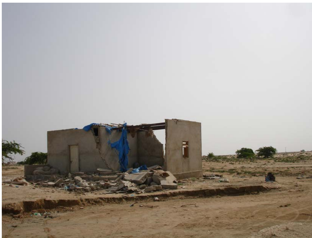
Figure 8: Some buildings are collapsed like this one. Photo credit: Ahmad Khan, PWP
